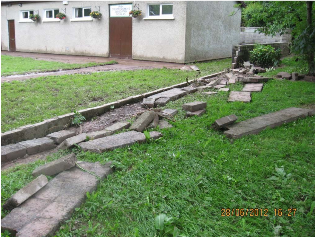
Figure 8.6: Post 2012 flood event – wall knocked down outside ICA Hall
