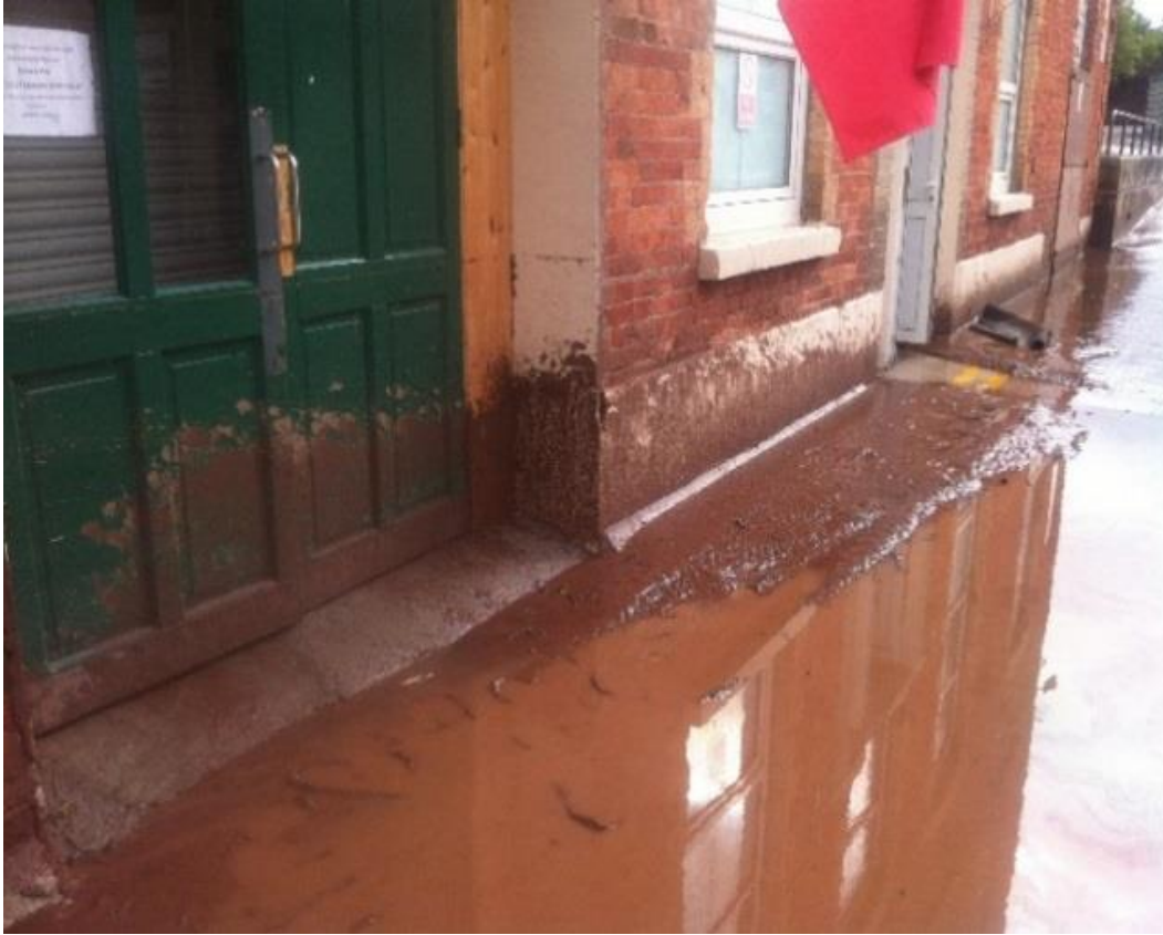
Figure 2.14: Post 2012 flood event at Donnybrook Commercial Centre. Source: Donnybrook Commercial Centre
